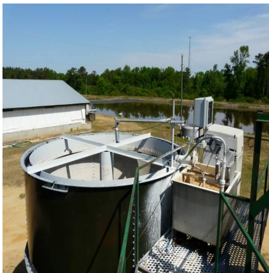
Illustration of liming for phosphorous removal in Tyndall Farm (North Carolina, USA)
