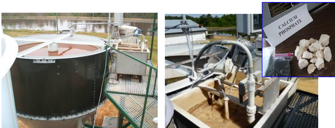
Illustration of the calcium phosphate precipitation unit at Tyndall Farm (South Carolina, USA). Detail of the CaO mixing chamber and of the final product obtained (see section 4.2)
