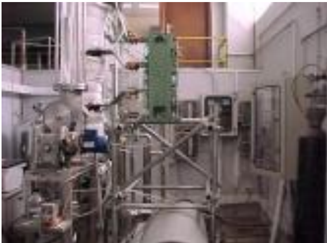
Illustration of a gasification pilot plant of the CEPIMA research group at UPC-BARCELONATECH ( http://www.upc.edu/pct/es/equip/297/planta-piloto-gasificacion-limpieza-gases-calientes.html )
