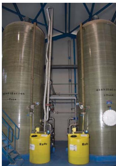
Ozonizing units at Alhama de Murcia (Murcia, Spain) pig manure treatment plant, OTSI technology (Infoenviro July/August 2008)
